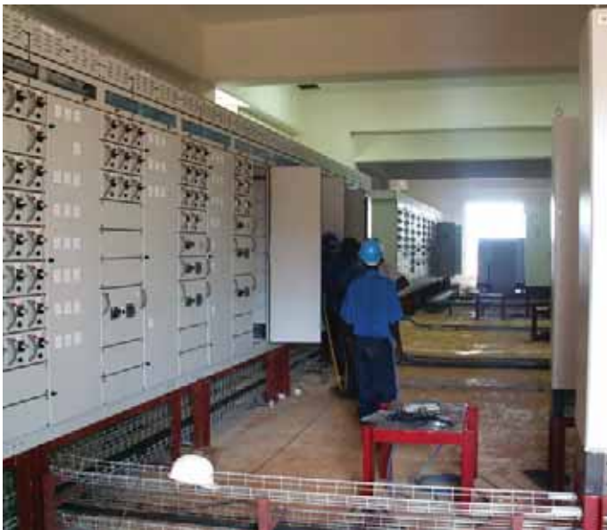
Low voltage electrical room
