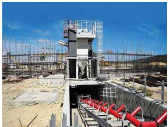
Extraction Belt conveyor from storage
